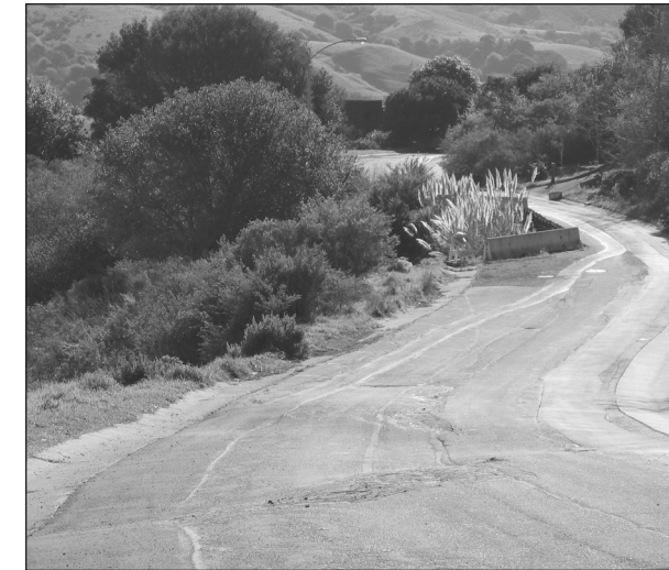
The unstable land in Canyon Estates. A house went down the hill in this area in 1983. Where Wildcat Drive slid out 10+ years ago is obvious toward the rear of this photo and in the foreground the road can be seen slumping as well.
